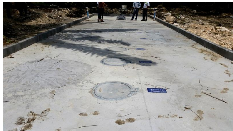
Wastewater treatment system at housing site.
