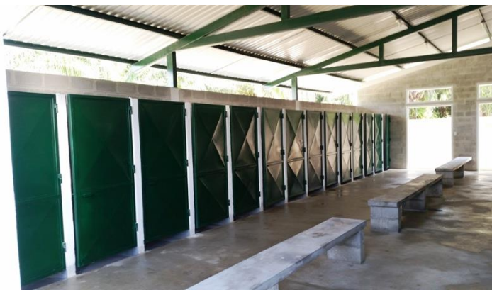
New worker showers at the "Union B" worker housing site.
