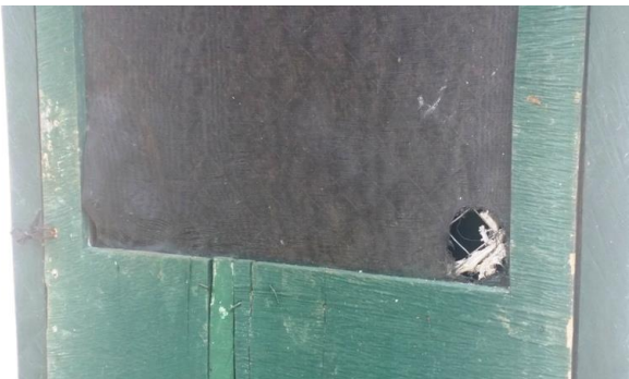
Figure __. Doors at housing sites require new locks that allow locking from inside and outside and mending of mosquito screens.
