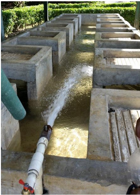
Filtered water at worker laundry area.
