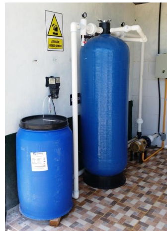
New water filtration for wash areas.
